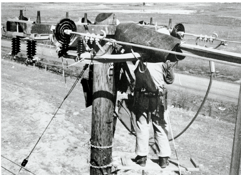
BELOW: A redesigned distribution system allowed linemen to work on energized lines. Note the insulation wrapped around the conductive surfaces in this photo.
