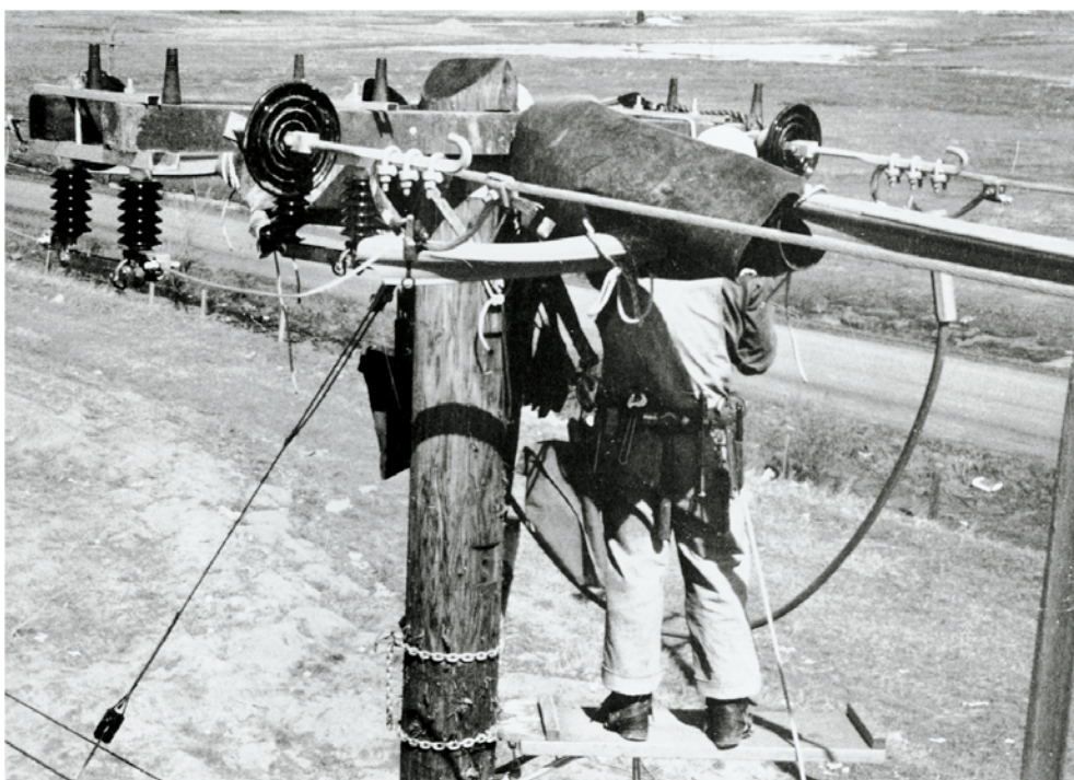
BELOW: A redesigned distribution system allowed linemen to work on energized lines. Note the insulation wrapped around the conductive surfaces in this photo.
